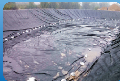
土工膜-蓄水池 Geomembrane Lined Reservoir
